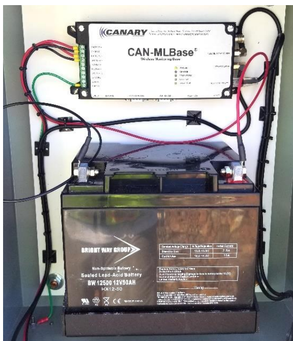
A correctly wired battery installed in an MLBase enclosure
